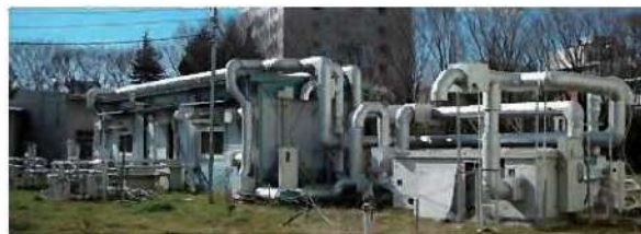
Experimental facility for testing a desiccant air-conditioning system combined with a heat pump (Institute of Industrial Science at the University of Tokyo)
