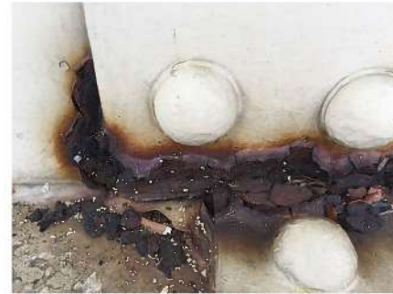
Corrosion deterioration due to chloride anti-freezing agents on a steel bridge
